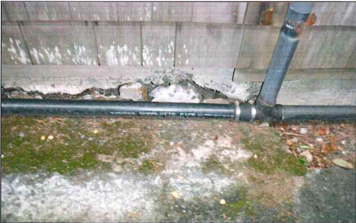
Photo 4 – Detail view of possible settlement or subsidence of existing foundation grade on north side of existing home, possibly due to past stormwater leakage into foundation soils.
