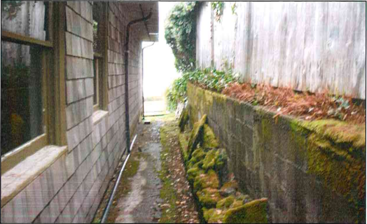
Photo 3- View to west beside north side of existing home showing adjacent retaining wall to north.
