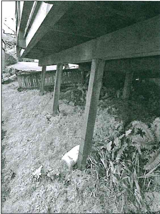
Figure 8: Tipping deck posts caused by downslope movement of shallow soils on steep slopes that are as steep as 90 percent, generally dropping at least 5 ft vertically over 7 ft horizontally (70 percent). The new deck footings will be on ground that drops 5 ft over 10 ft (50 percent) or less.
